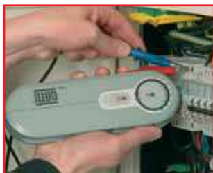
Picture of installation without presence voltage.
